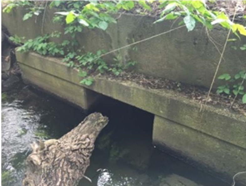
48"x48" Open Bottom Box Culvert (Upstream) – Condition observed to be adequate and structurally sound
