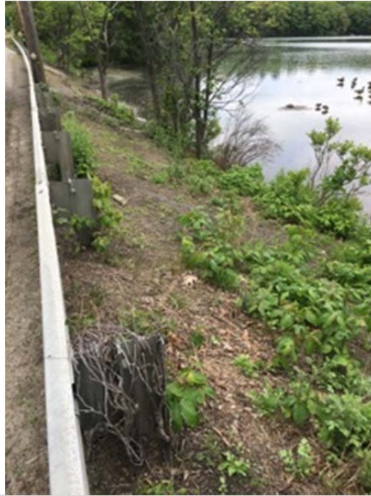
Slope on south side of Route 20 along Hager Pond, east of culvert crossing
