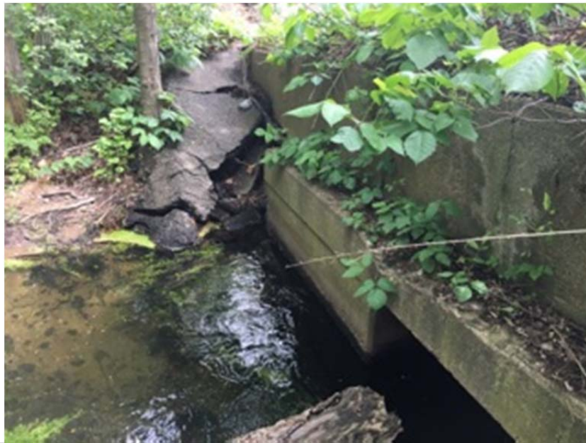
Upstream box culvert – broken paved swale from Route 20
