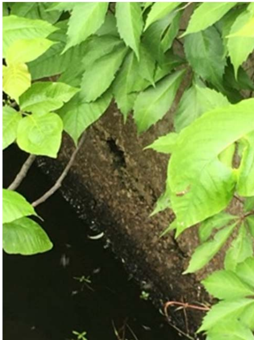
Small crack in downstream headwall (approximately 18" in length)
