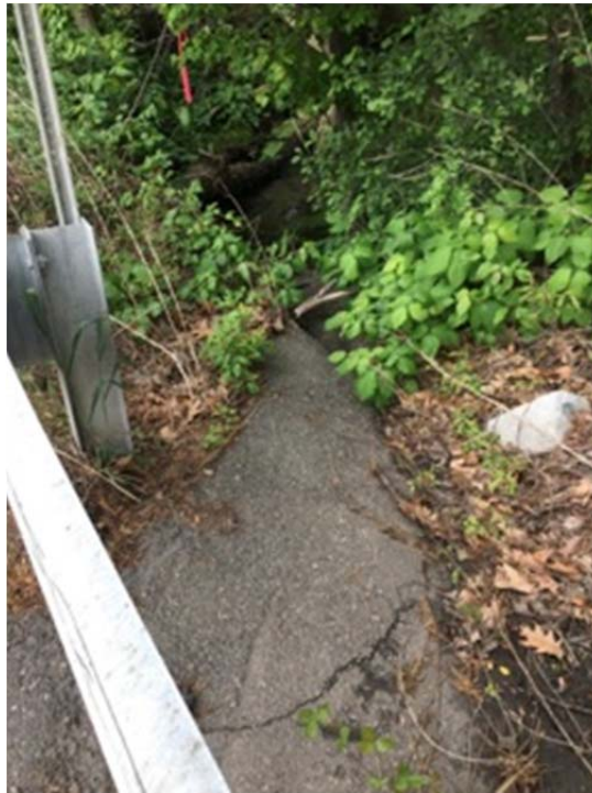
Broken paved swale from Route 20 – upstream box culvert
