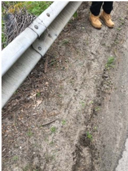
South side Route 20 sediment build up to guard rail
