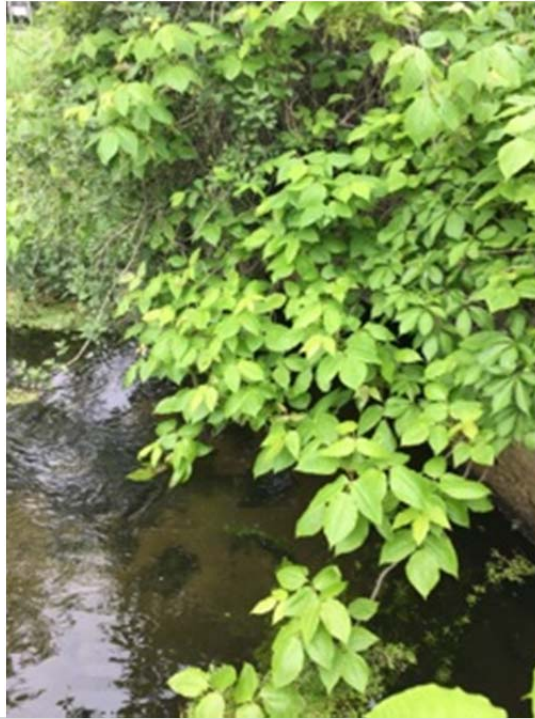
Downstream culvert (Hager Pond outlet) – overgrown vegetation
