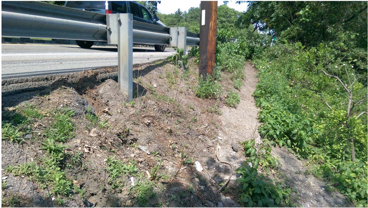
Eroded Slope on south side of Route 20 along Hager Pond, east of culvert crossing
