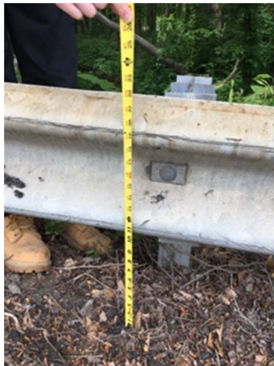
Upstream box culvert – guardrail height approximately 22"
