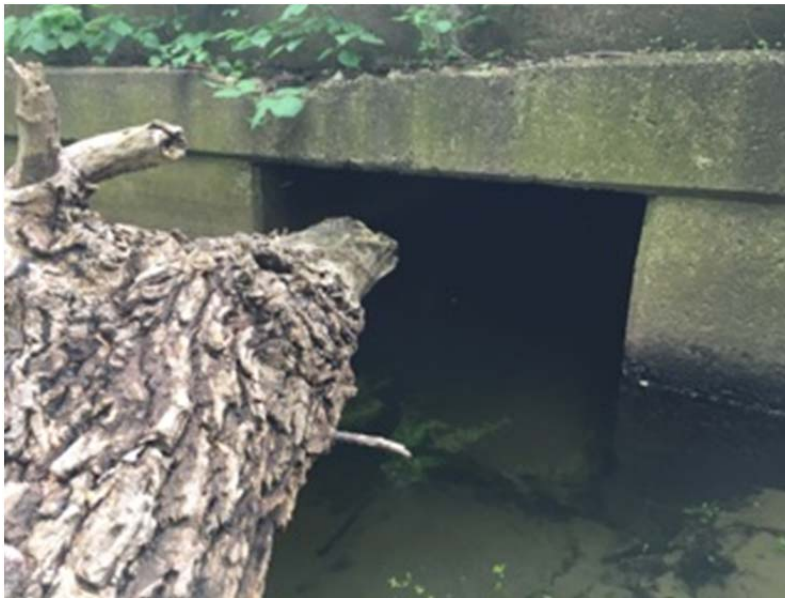
Looking down box culvert upstream – from what could be seen, inside of culvert looks structurally sound
