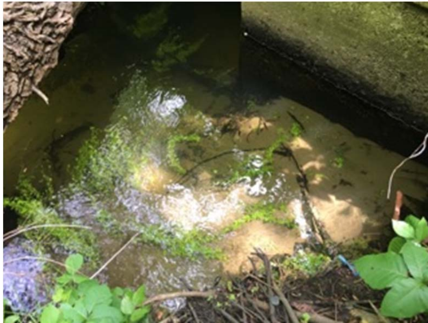
Approximately 18" built up sediment upstream side of box culvert, water level approximately 30" depth
