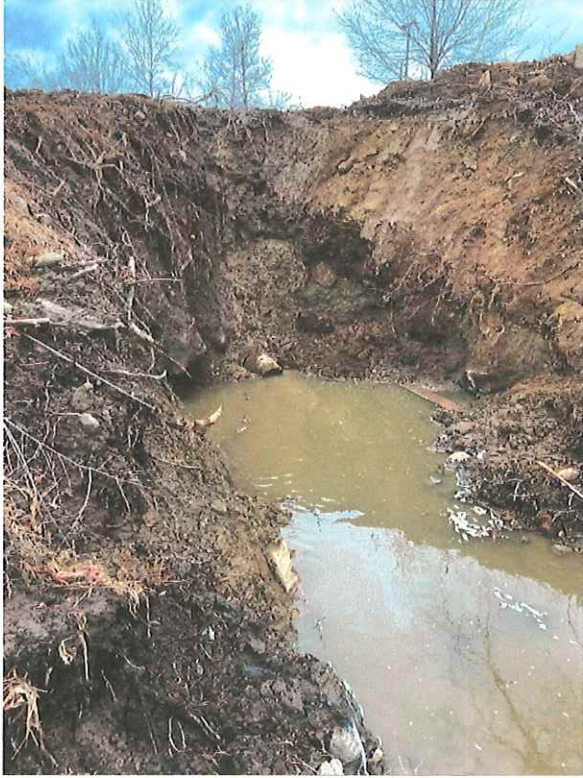
Downstream pipe exposed, and slopes completely unstable.
