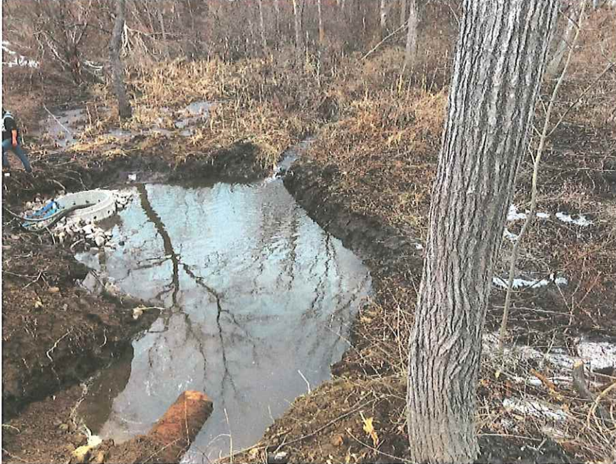
Upstream of drainage culvert- see corrugated inlet pipe at bottom of photo
