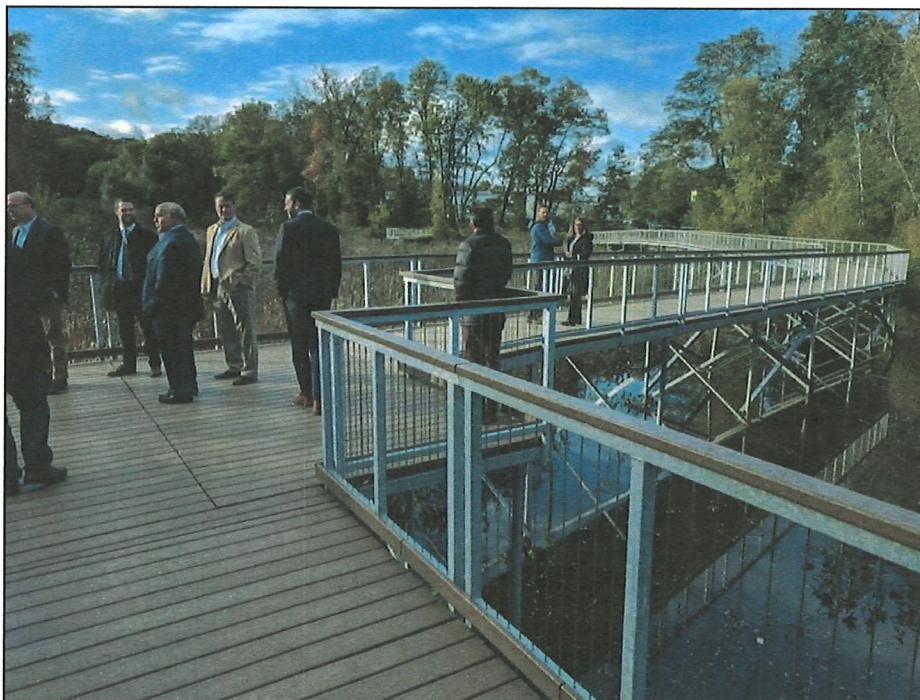
Photo 2: Boardwalk Project at Middle River Park, Worcester. Helical piles with supporting crossbeams visible in background. Source: Grant Welker/Worcester Business Journal
