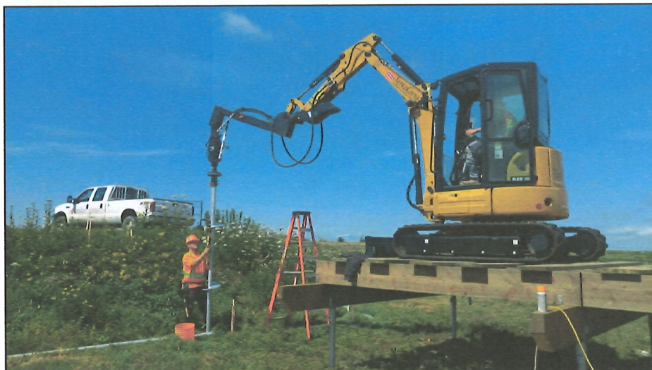
Photo 4: Boardwalk constructed with small, tracked machine driving helical piles.. Source: TerraCana Foundation Solutions, Inc.
