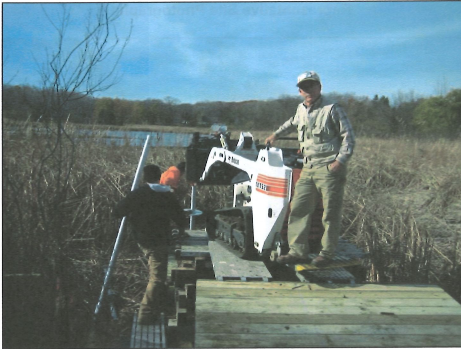
Photo 3: Helical piles being installed using machine on constructed boardwalk in wetland. Source: Foundation Support Systems
